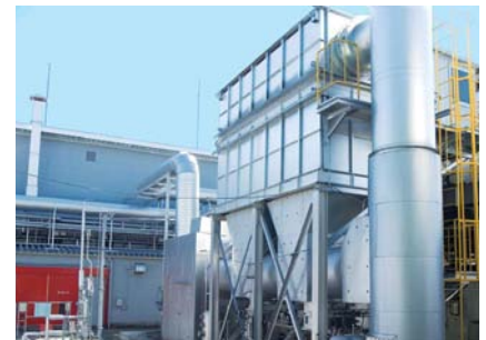
Exhaust-gas treatment facility
