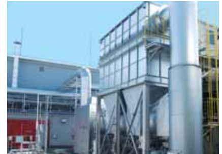
Exhaust-gas treatment facility
