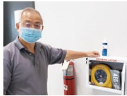
Installed AED device
