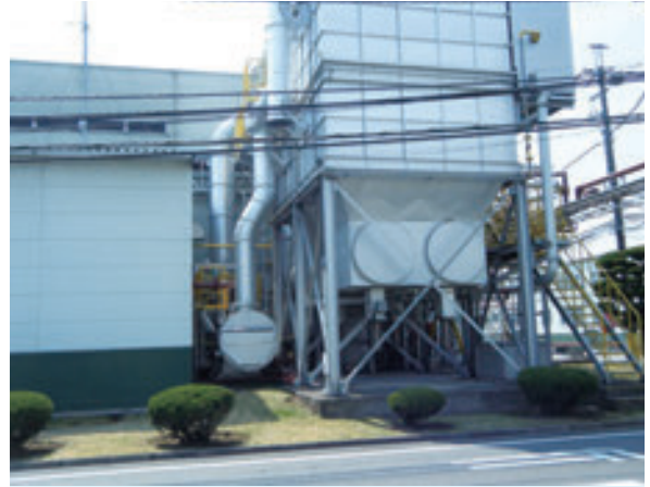
VOC waste heat recovery boiler at the Kumagaya Plant
