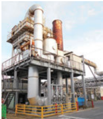
Waste heat boiler at the Chiba Plant
