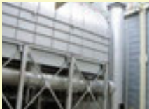
VOC heat incineration system
