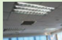
LED lighting in the office
