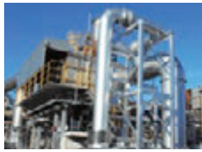
Waste-heat boiler installed in the Chiba Plant
