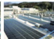
Solar panels at the Agatsuma Plant (about 5,000 m 2 )
