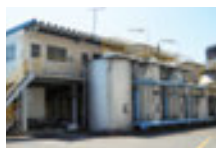
Effluent processing equipment at the Mishima Plant
