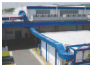
Exhaust duct for air conditioning air
