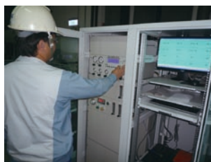
Automatic VOC monitoring device
